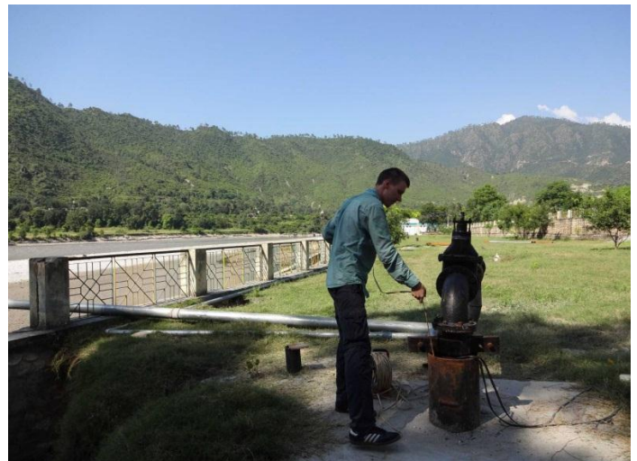
Figure 3: Monitoring well 5 constructed in Srinagar in between the Alaknanda and PW5 (right), on which a pumping test is being conducted.
