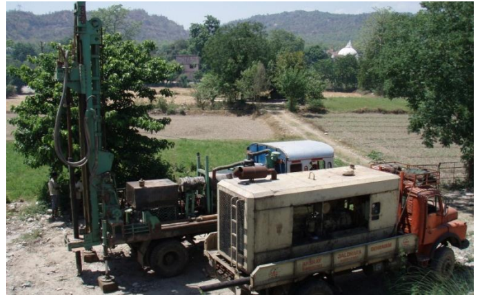
Figure 1: Construction of monitoring wells at the bank filtration site in Haridwar by Akshay Jaldhara (Photo: K. Heinze & M. Lesch, HTWD, May 2012)
