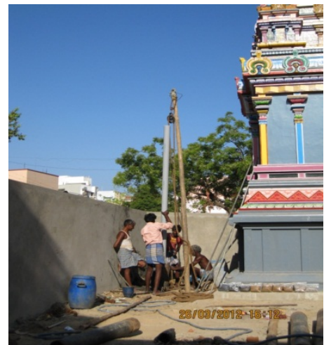
Construction of observation borewell (hand bore) near Agatheeswarar Temple Tank – lowering of casing pipe in progress
