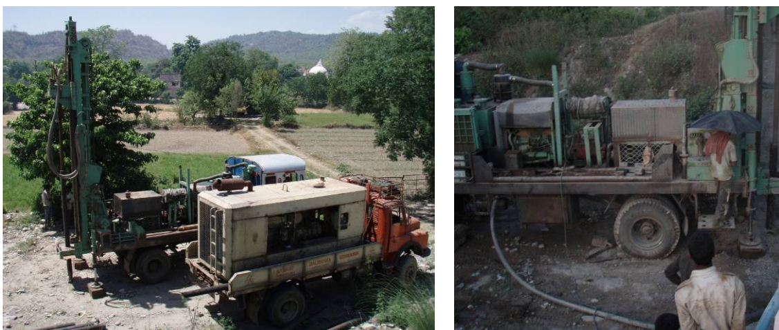
Figure 4-1 Construction of monitoring wells at the RBF site (IW2) in Haridwar by Akshay Jaldhara (Photo: K. Heinze & M. Lesch, HTWD, May 2012)
