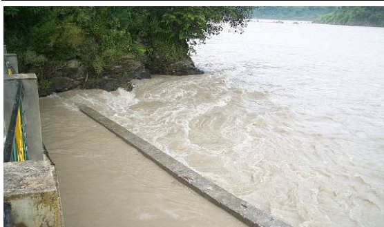
Figure 3-3 Intact retaining wall at the downstream-end of the RBF site in Srinagar at the onset of the monsoon flood in August 2011 (Photo: J. Ebermann, HTWD, 2011)
