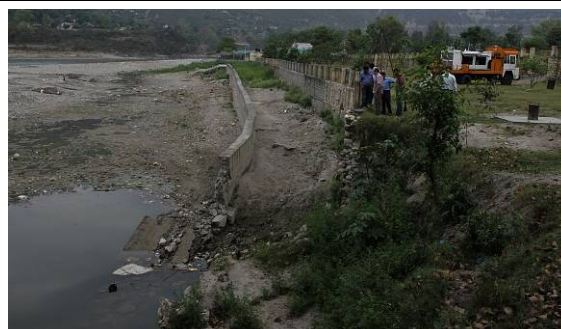
Figure 3-4 Damaged retaining wall of the RBF site in Srinagar after the monsoon flood of August 2011 (facing upstream) (Photo: T. Voltz, HTWD, 2012)
