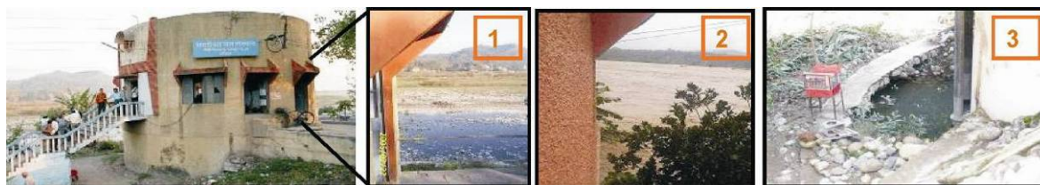
Figure 2-6 RBF well IW 24 in Haridwar (left photo), (1) view of the Ganga River in the background in April 2005 (pre-monsoon), (2) flood-water of Ganga inundates the base of well on 19/09/2010 and (3) damage by scouring to base of well no. 24 (photos from L to R: Schoenheinz and Grischek (2005), Subodh & Kumar (2010))
