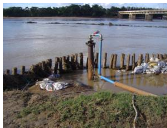
Figure 3-6 A RBF well in Kharagpur (Kangsabati River, West Bengal) at risk of contamination by floods (Photo: C. Sandhu)
